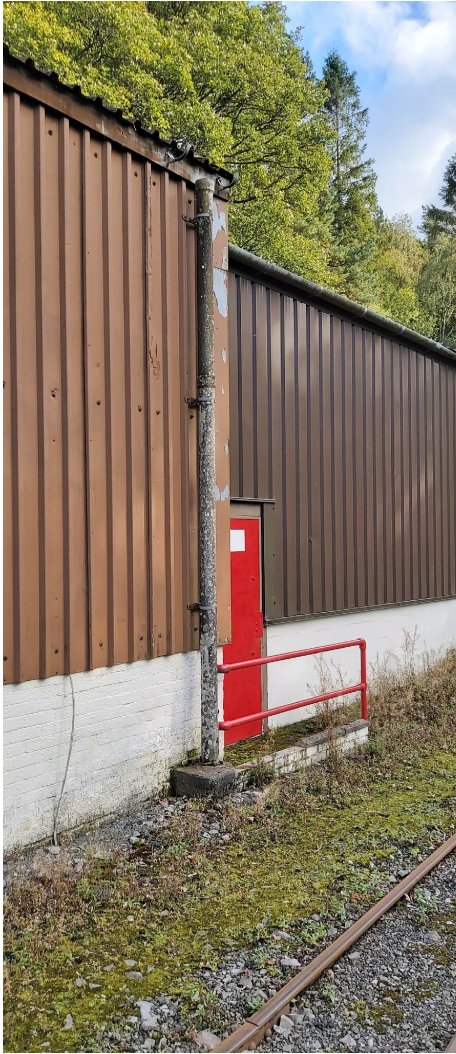
2020 Asbestos Survey – Photograph – Ref: Zer/st/ry/11 Location Ref: AS05 Location: Ground Outside Shed 2
