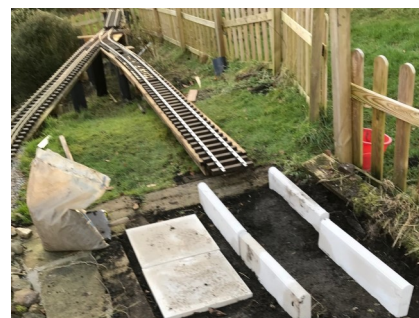
The spur to the new loco shed (Shed 52d!) should be finished by half term.
